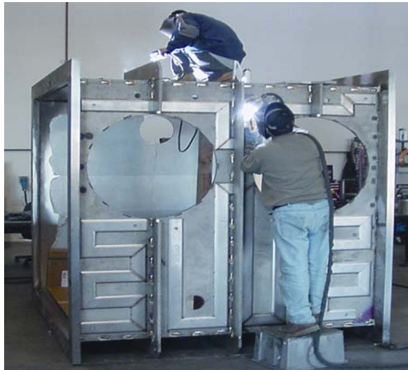
Fig 4: This box chamber is covered with water traces to provide cooling.
